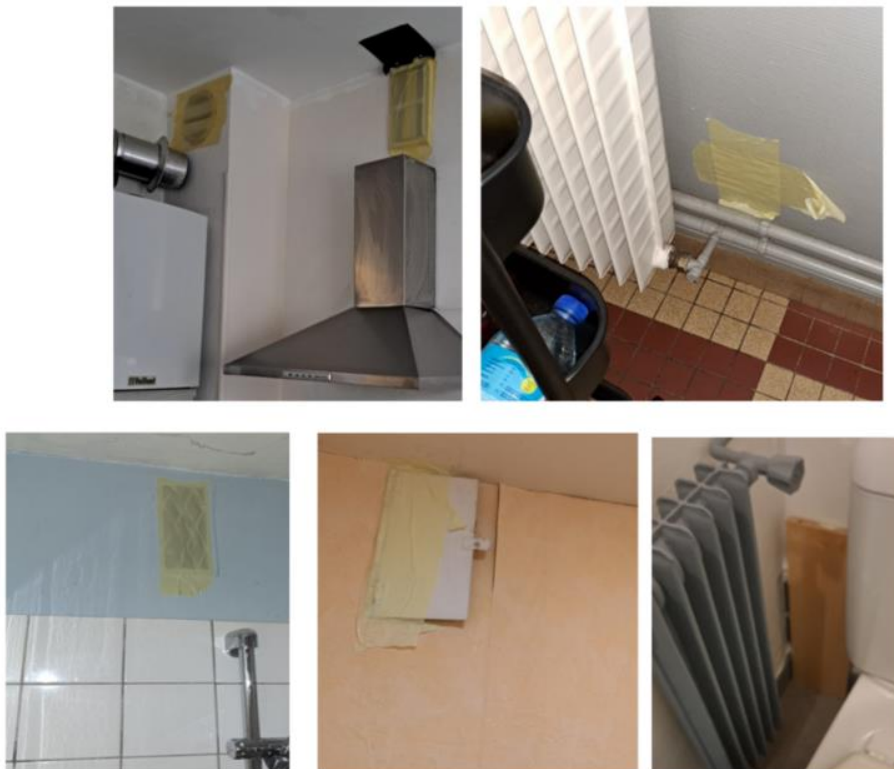
Figure 31: natural air inlet grilles and boiler smoke exhaust
