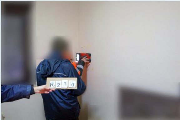
Figure 95: Georadar survey of reinforcement bars at column 21 on the upper ground floor, flat interior.
