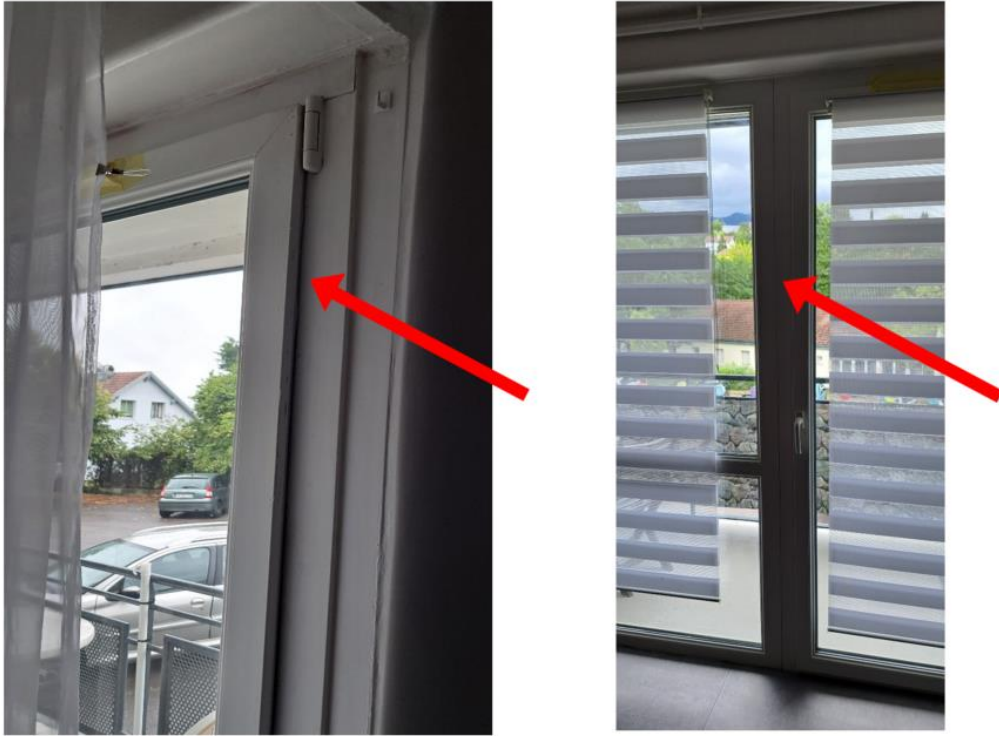
Figure 26: deformation of the sash on the living room French window, creating a gap that the seal no longer covers. joinery seal between living room window and French window
