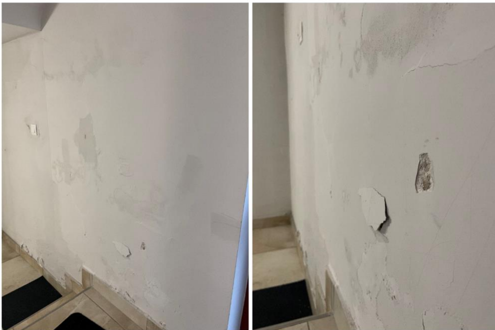
Figure 22: Wall watering in the corridor
