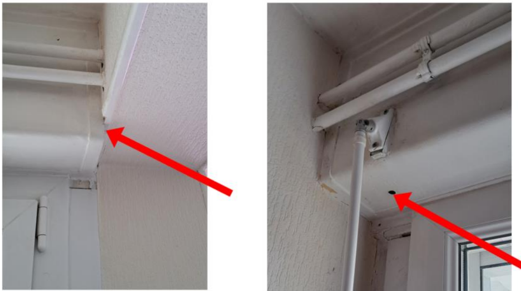
Figure 27: leak at connection in living room. A hole in roller shutter box. Leak in the roller shutter mechanism
