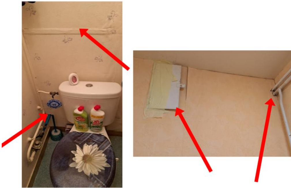
Figure 30: bushings, fittings, natural air extraction
