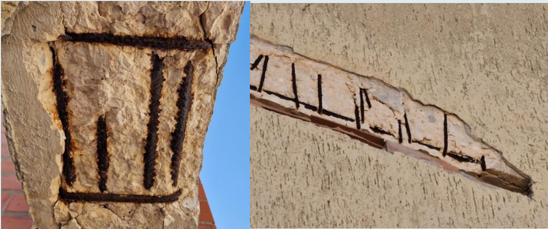
Figure 81: Degradation of concrete and corrosion of the reinforcements.
