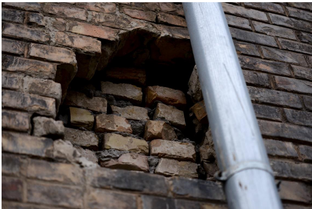
Figure 24: Defect on the exterior brick façade. Original bricks are missing in several places
