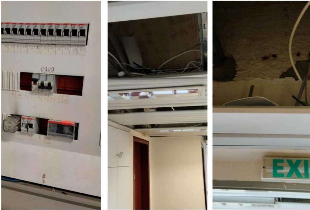
Figure 45: Fuses at the Electrical Panel(RH), Raspberry Pi and Router installation
