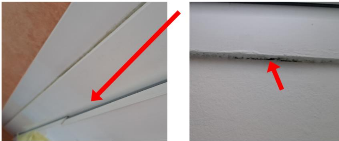
Figure 29: Air intake at top/bottom sash connection. Two windows no longer close properly
