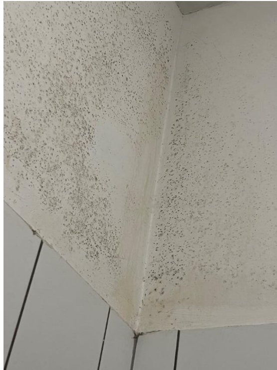
Figure 23: Molds on the wall surface especially in the corners in the bathroom
